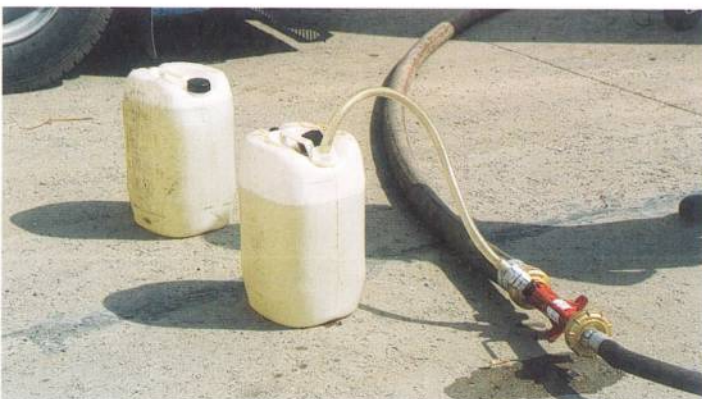
3.15 Using an in-line inductor and foam concentrate in 25-litre drums. At 200 l/min and a 3% foam concentrate mixture, a 25-litre drum will last a good four minutes.
