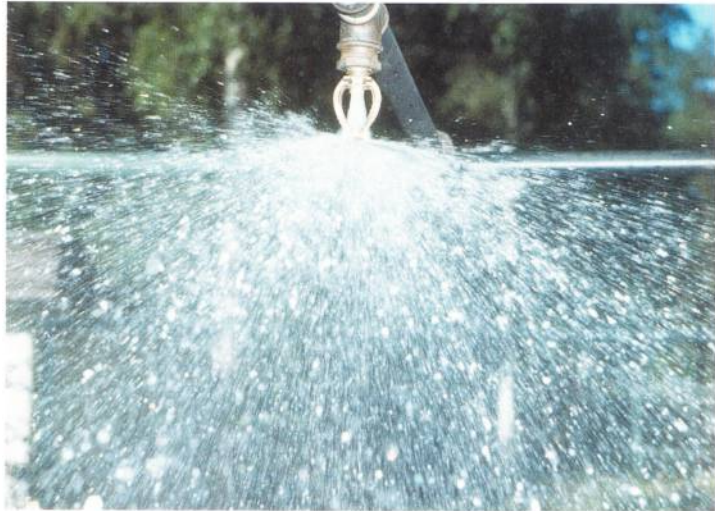
2.97 Activated sprinkler head.
