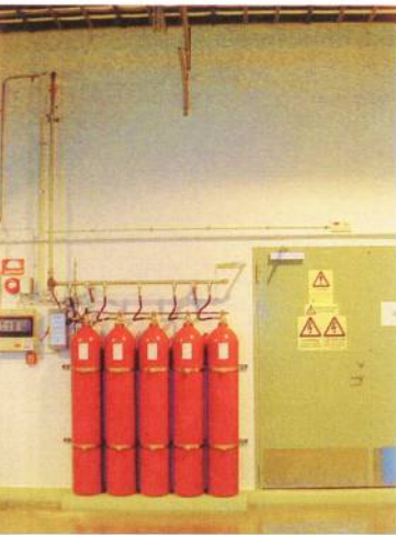
5.6. Fixed carbon dioxide installation protecting a room containing vital electronics.
