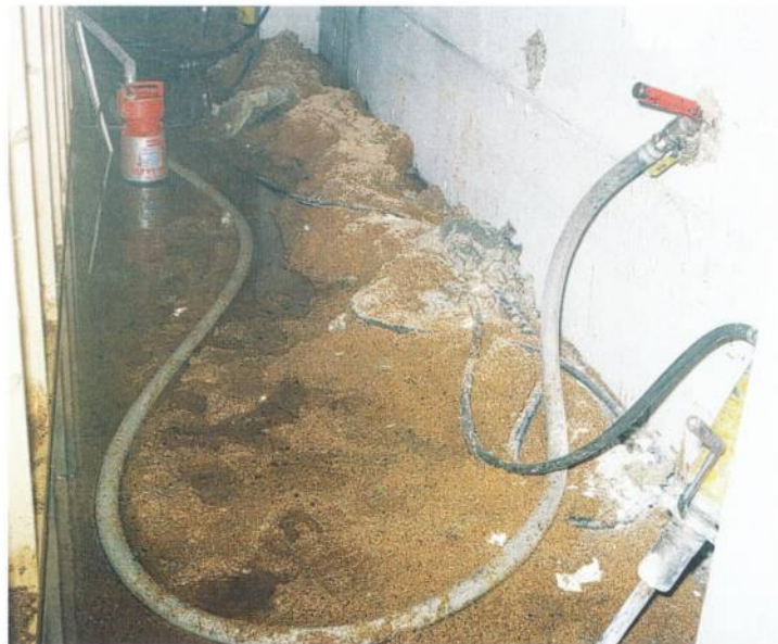
2.122 By drilling a hole in the wall (the drill is on the right) and inserting a piercing nozzle, the heat impact on the fire wall is reduced.
