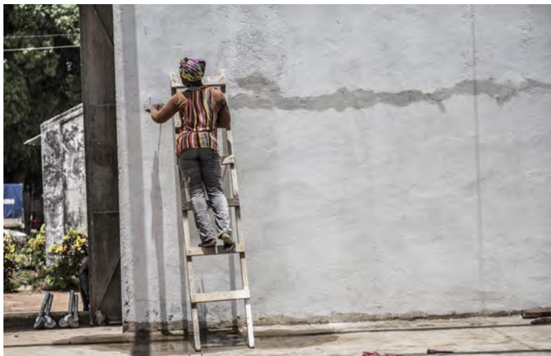
Contracted local female worker is carrying out renovation work of an office and accommodation compound in Bouar in CAR. Photo: Johan Lundahl, MSB, 2017
