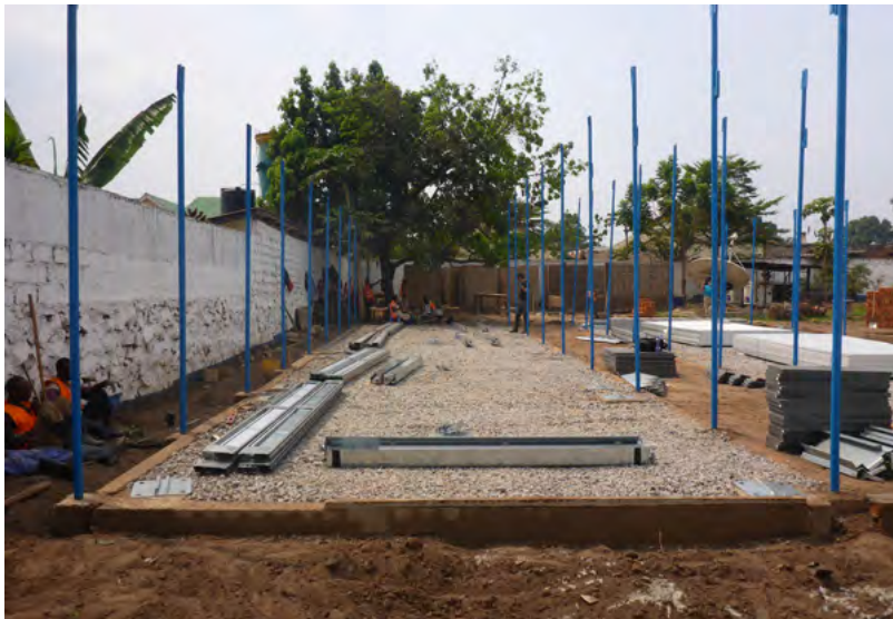
Contracted local female and male workers are taking a break in the shadow from the construction of a number of office and accommodation facilities for WFP in Kananga, DRC. Photo: Kerstin Degerman-Oldgren, MSB, 2018.
